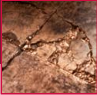
SLAB CORNER BREAKS
