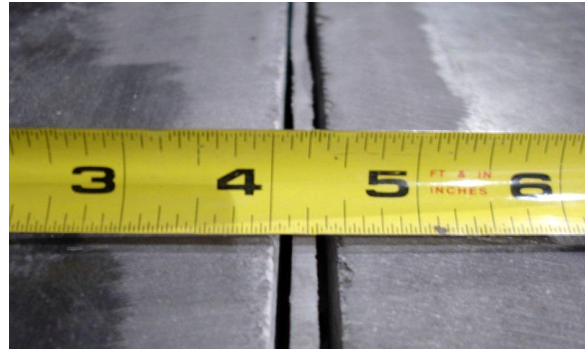
Right: Example of filler collapse in joint experiencing substantial opening...
