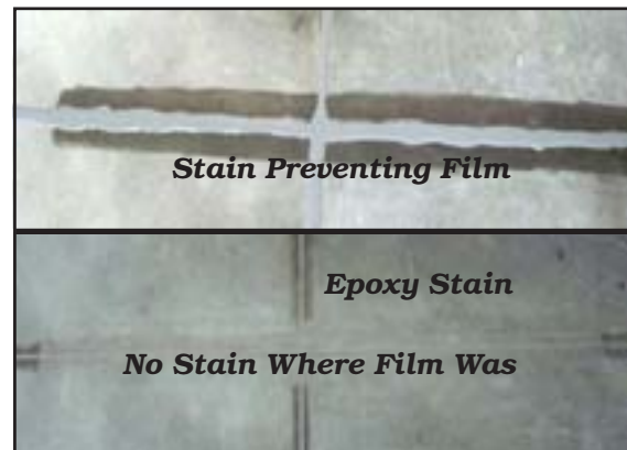
The use of a stain preventing film can reduce or eliminate slab surface staining from epoxy/polyurea filler overfill. Other stain prevention methods include applying soap or wax.
