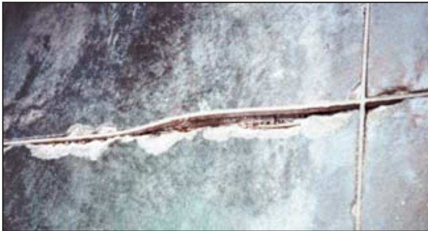
Improper filling of joints (in this case inadequate filler depth) is just one of many common causes of joint problems an owner may face, but it is one of the most easily preventable.
