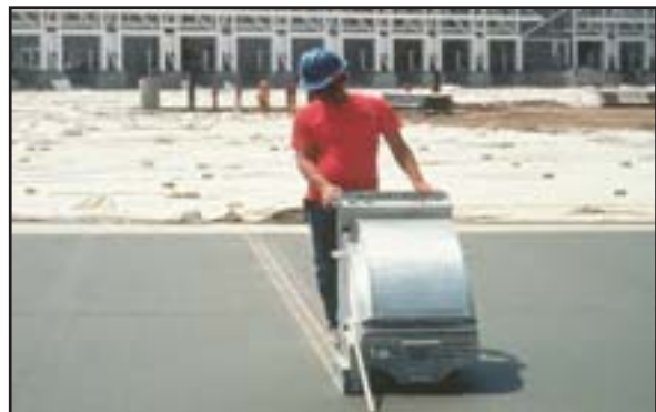
“Early Entry” saws allow for joint cutting to be performed within hours of slab placement, reducing the potential of random cracking and allowing for a shallower joint depth to induce cracking below the joint.
